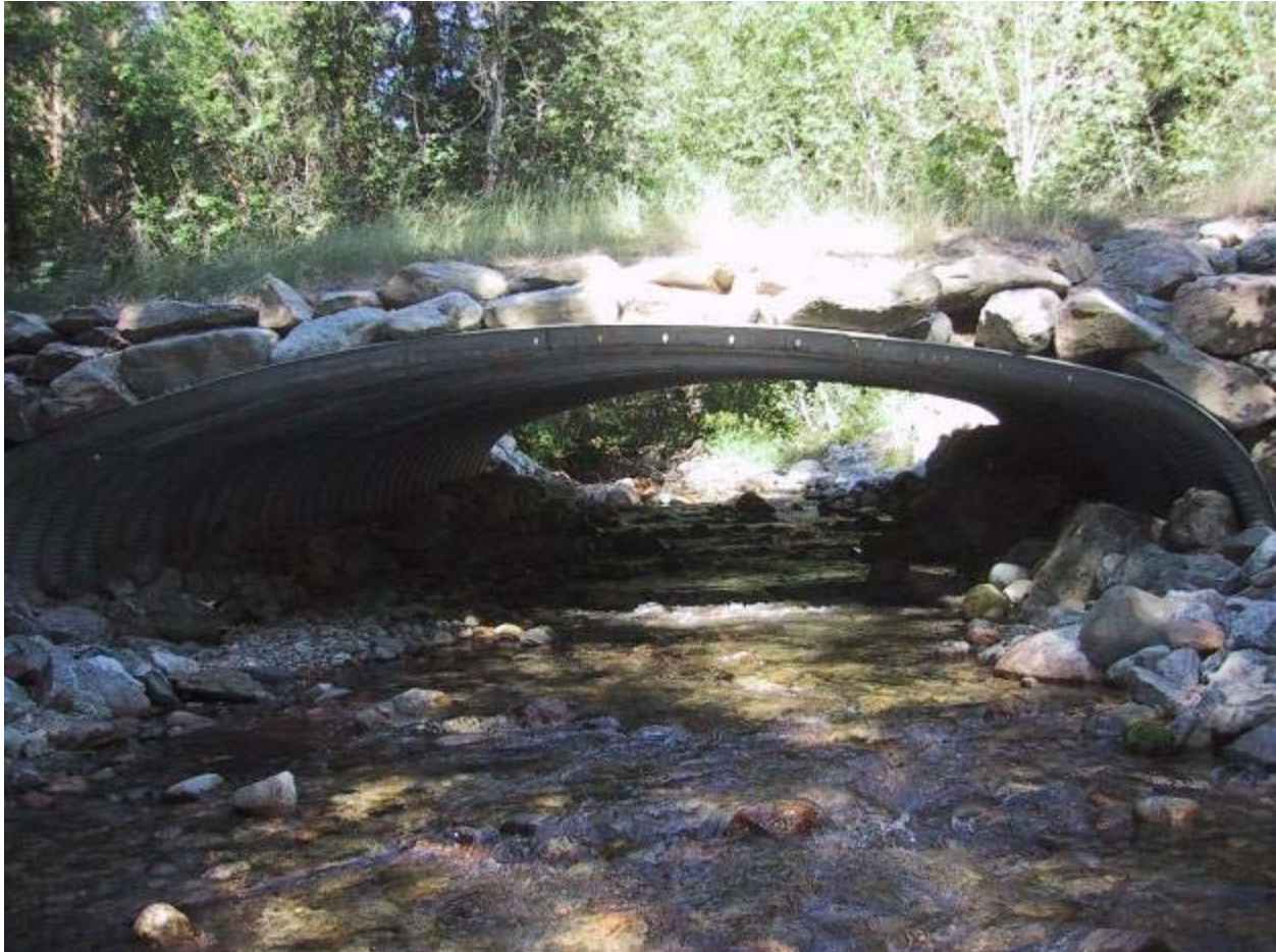
Figure XII-11. Stream simulation culvert in Twenty-Six Mile Creek, Washington State.
