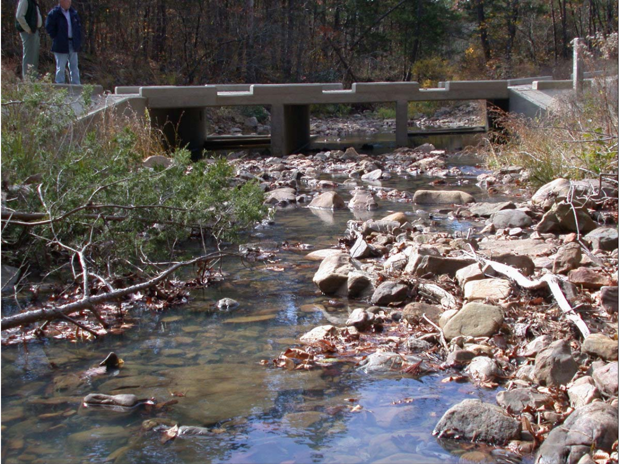
Figure XII-19. A vented ford constructed with three embedded concrete box culverts that span the bankfull channel and convey the bankfull flow without overtopping (FishXing Case Studies 2008).
