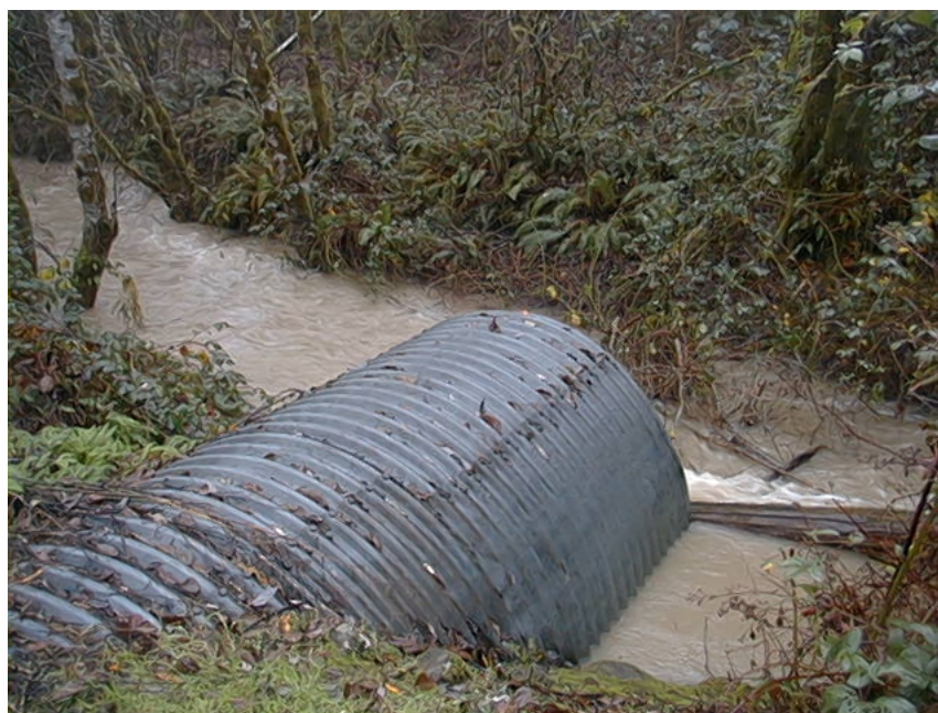
Figure XII-3. Poorly aligned culvert. Note log causing a blockage.
