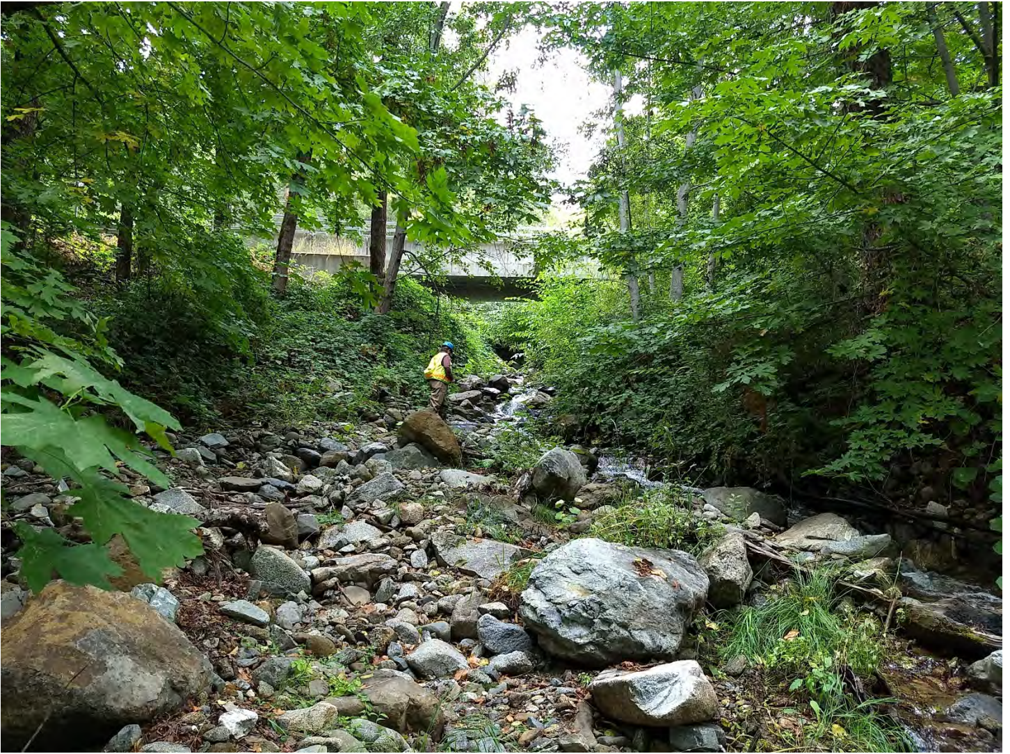
Figure 1. Channel downstream of the bridge looking upstream. Photo by M. Lang on 9/19/2019.
