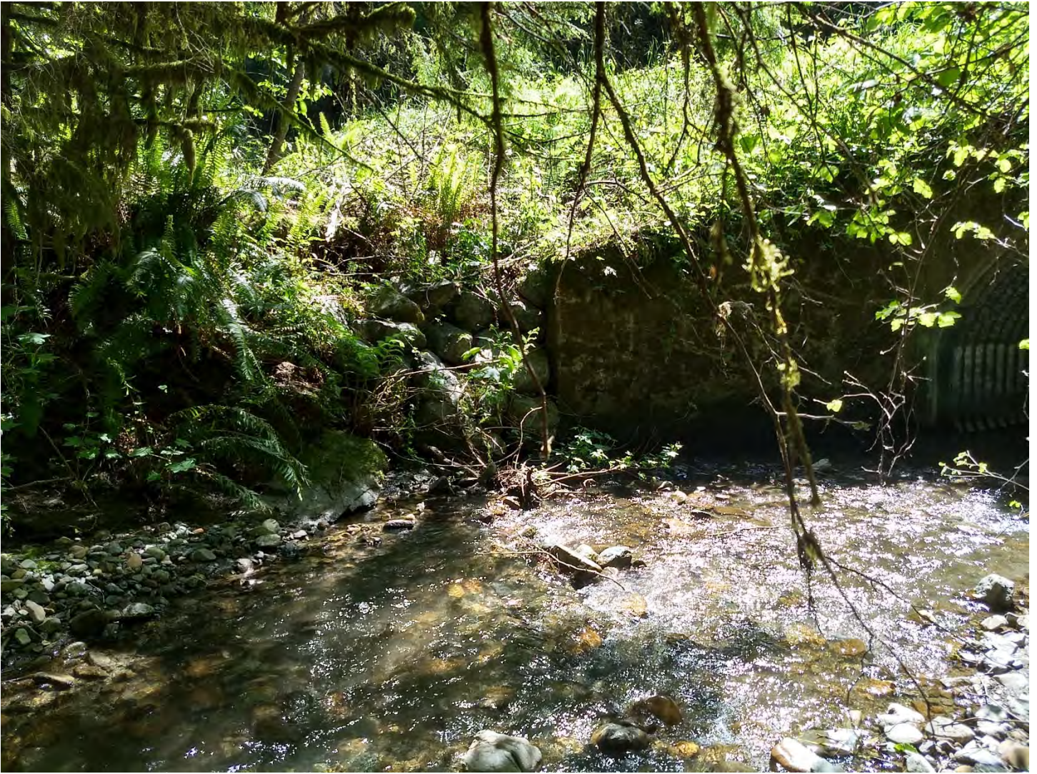
Figure 2. Left inlet wingwall showing some bank erosion from backwatering during high flows.
