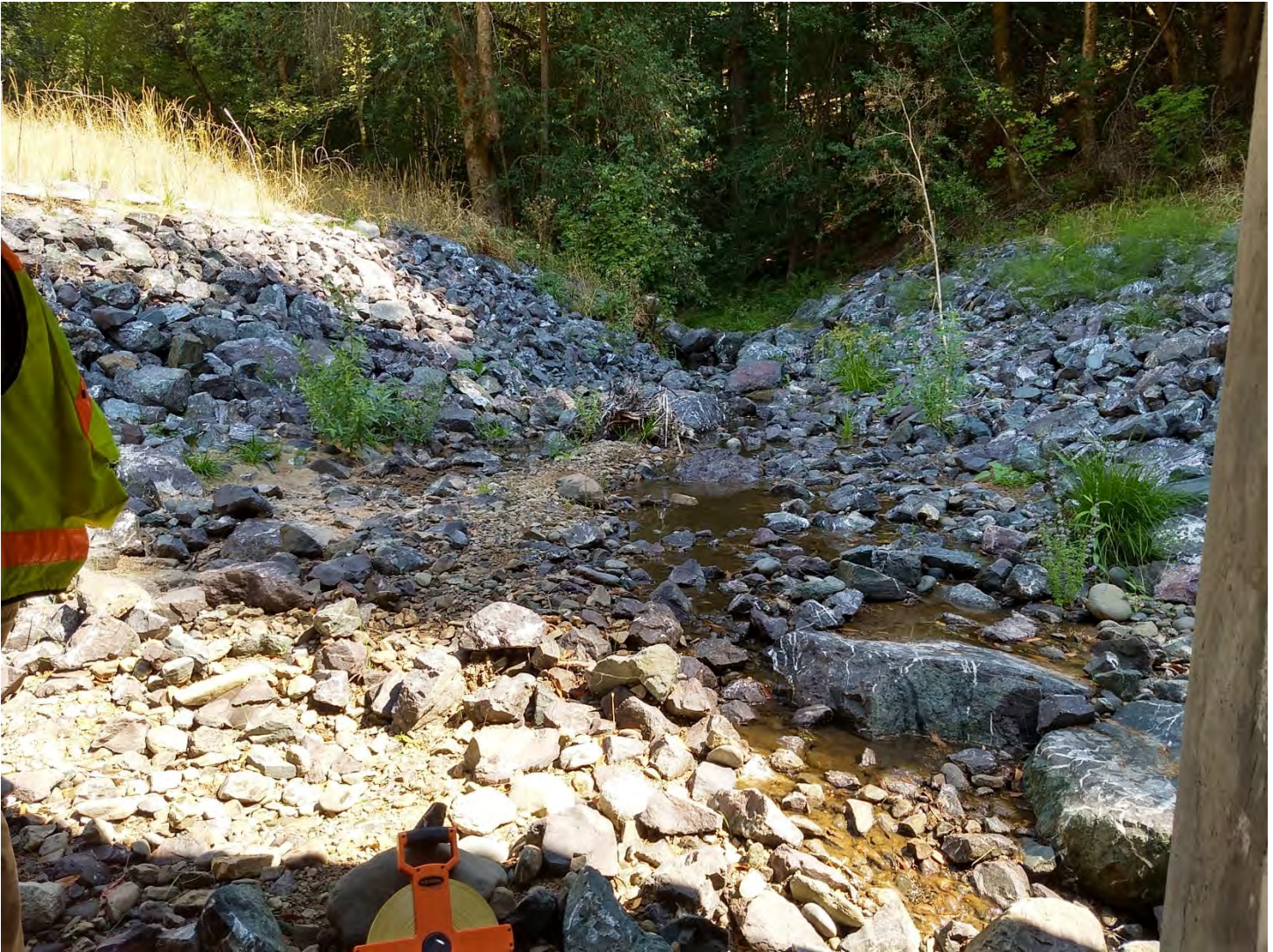
Figure 1. View looking upstream from the North Fork Ryan Creek culvert inlet. The rock weir installed for grade control at the upstream project boundary has a low flow drop of approximately 1.5 feet. Note that flow goes subsurface at the lower right corner of the photo. Photo by Margaret Lang on 9/12/2019.
