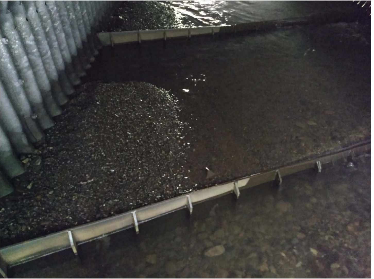
Figure 4. Sediment accumulation behind most baffles.
