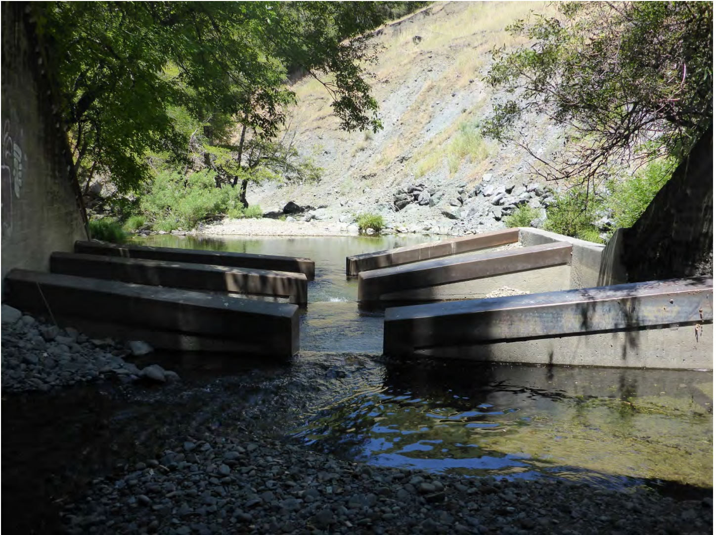
Figure 4. The outlet pool weirs and right channel bank looking downstream from the culvert outlet. The modifications to add the weirs and reorient the outlet flow away from the right bank has reduced the erosion of the right channel bank. Photo M. Love on July 17, 2019.
