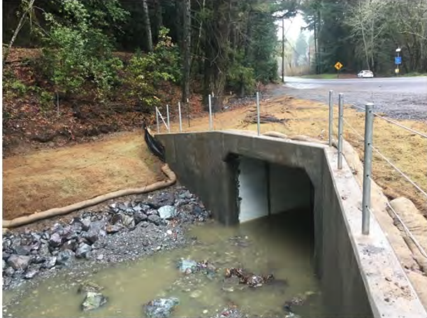
Culvert Outlet Post-Treatment. Photo taken on 01/09/2018 and courtesy of Caltrans.
