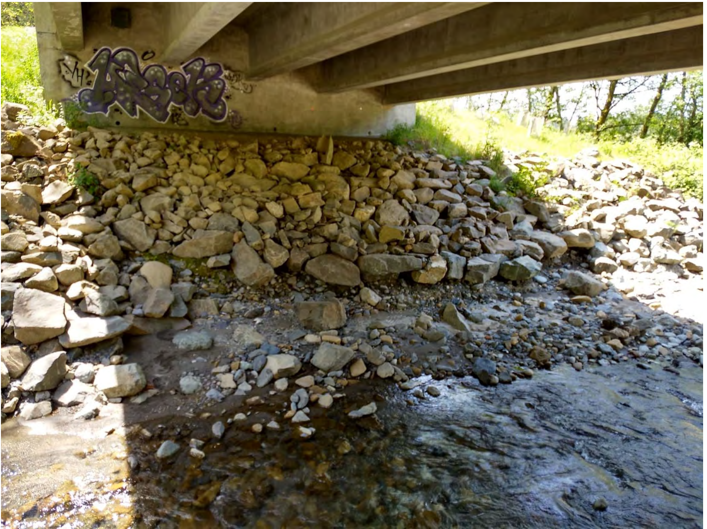
Figure 5. Left bank erosion of rip rap toe. Lowest rock appears to be missing.
