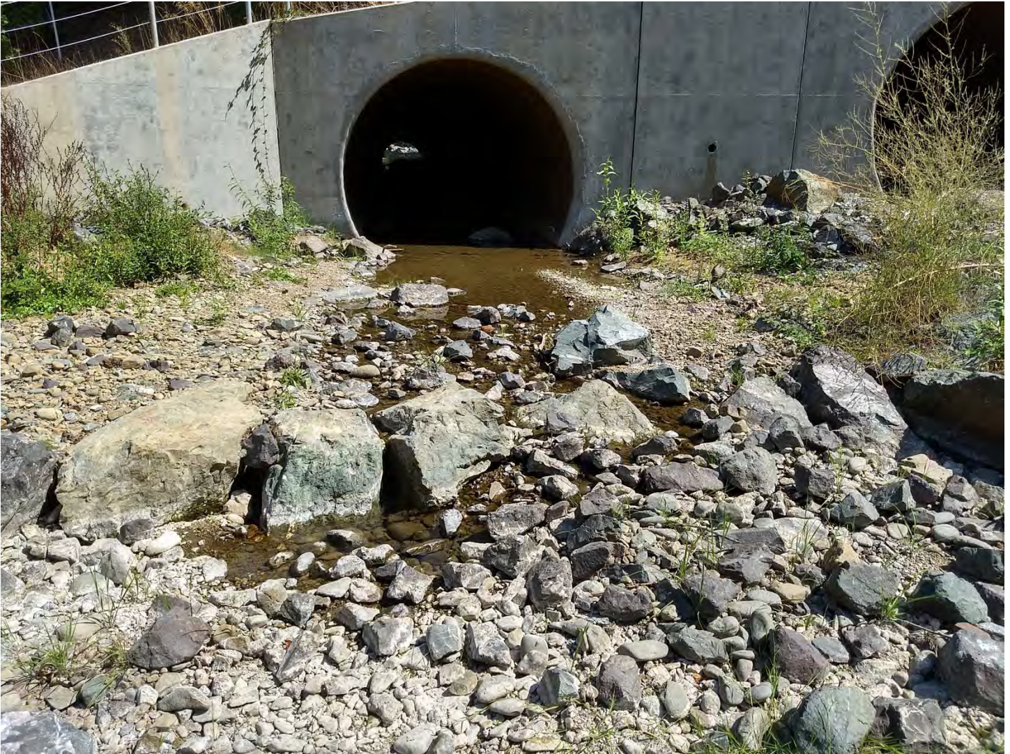
Figure 6. The lower culvert's outlet looking upstream. At low flows, the flow goes subsurface and was discontinuous starting at the first rock weir downstream as seen in the photo's foreground. Photo by Margaret Lang on 9/12/2019.
