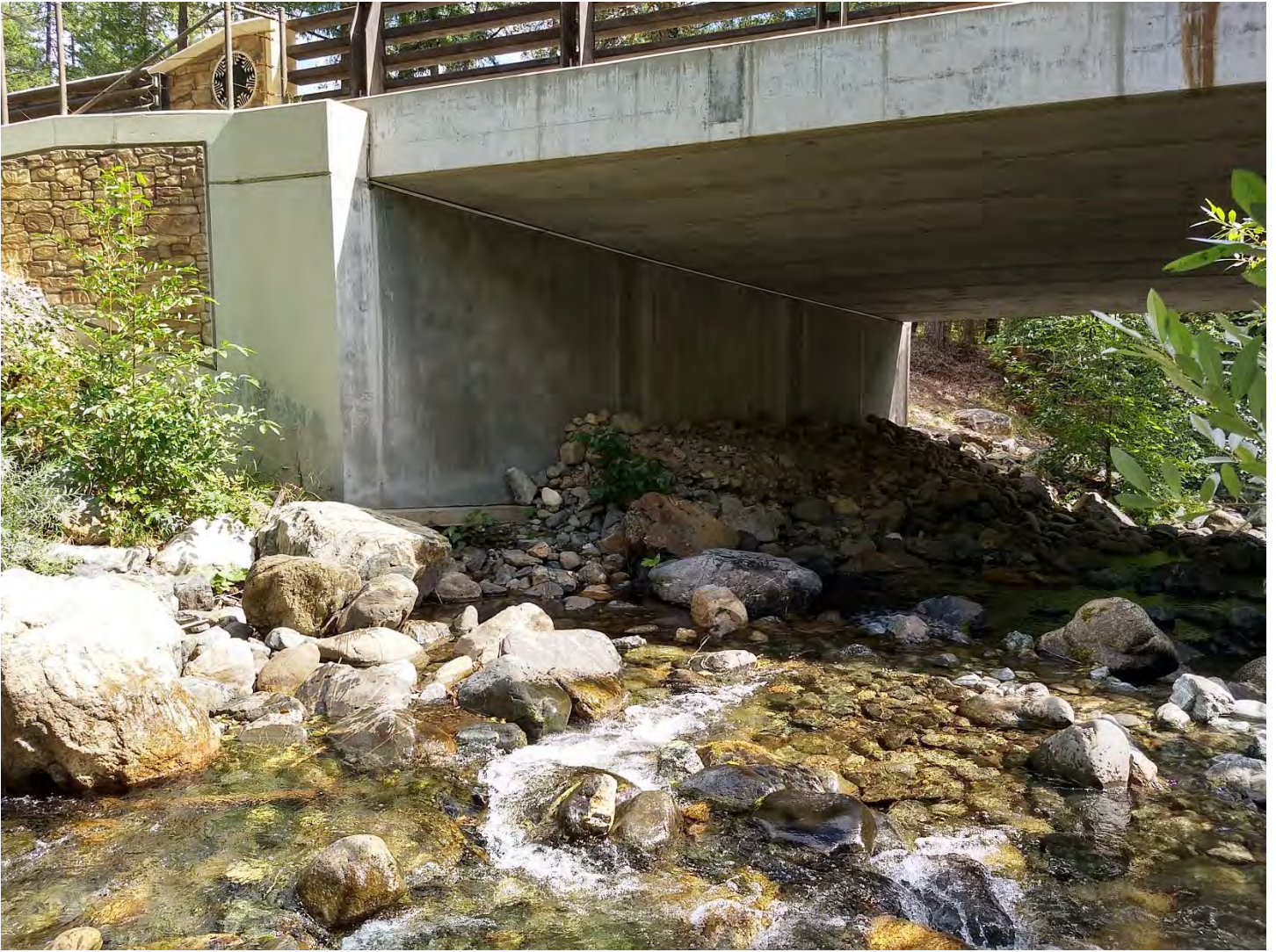
Figure 3. Upstream, left bank of bridge showing scoured bank protection and exposed footing. Photo by M. Lang on 9/19/2019.
