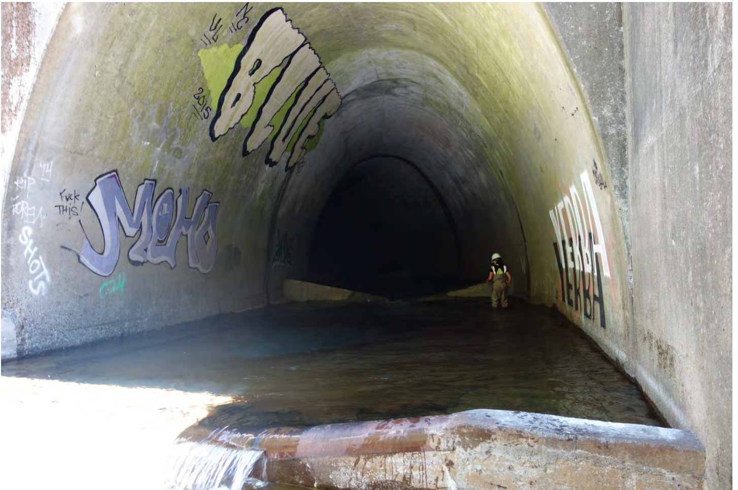
Figure 4. Cedar Creek culvert looking upstream from the outlet. The internal fish weirs are functioning well. Photo taken June 3, 2021.
