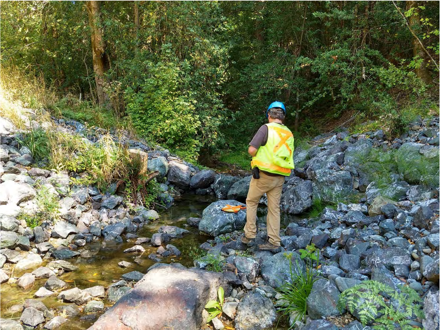
Figure 2. Close-up view of the upstream rock weir. The footing rocks are exposed in the pool increasing the potential for weir failure. Note that the low flow is going through the rocks in the weir rather than over the crest. Photo by Margaret Lang on 9/12/2019.
