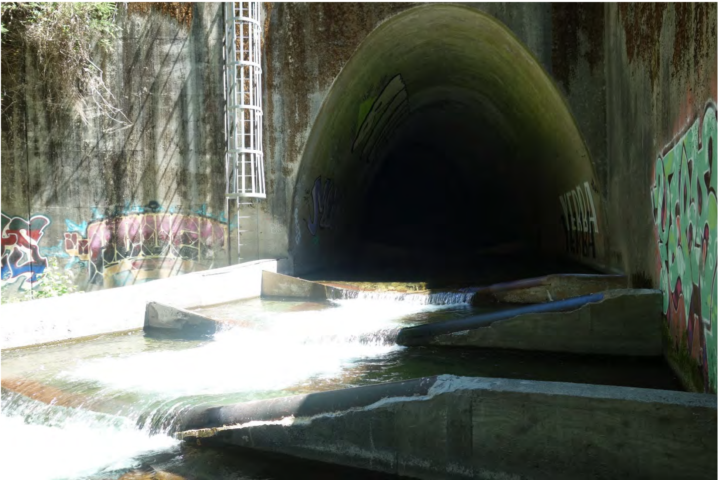
Figure 10. Cedar Creek culvert outlet weirs showing some of the crumbling concrete weir edges, especially around the installed steel plate coverings. Photo taken June 3, 2021.
