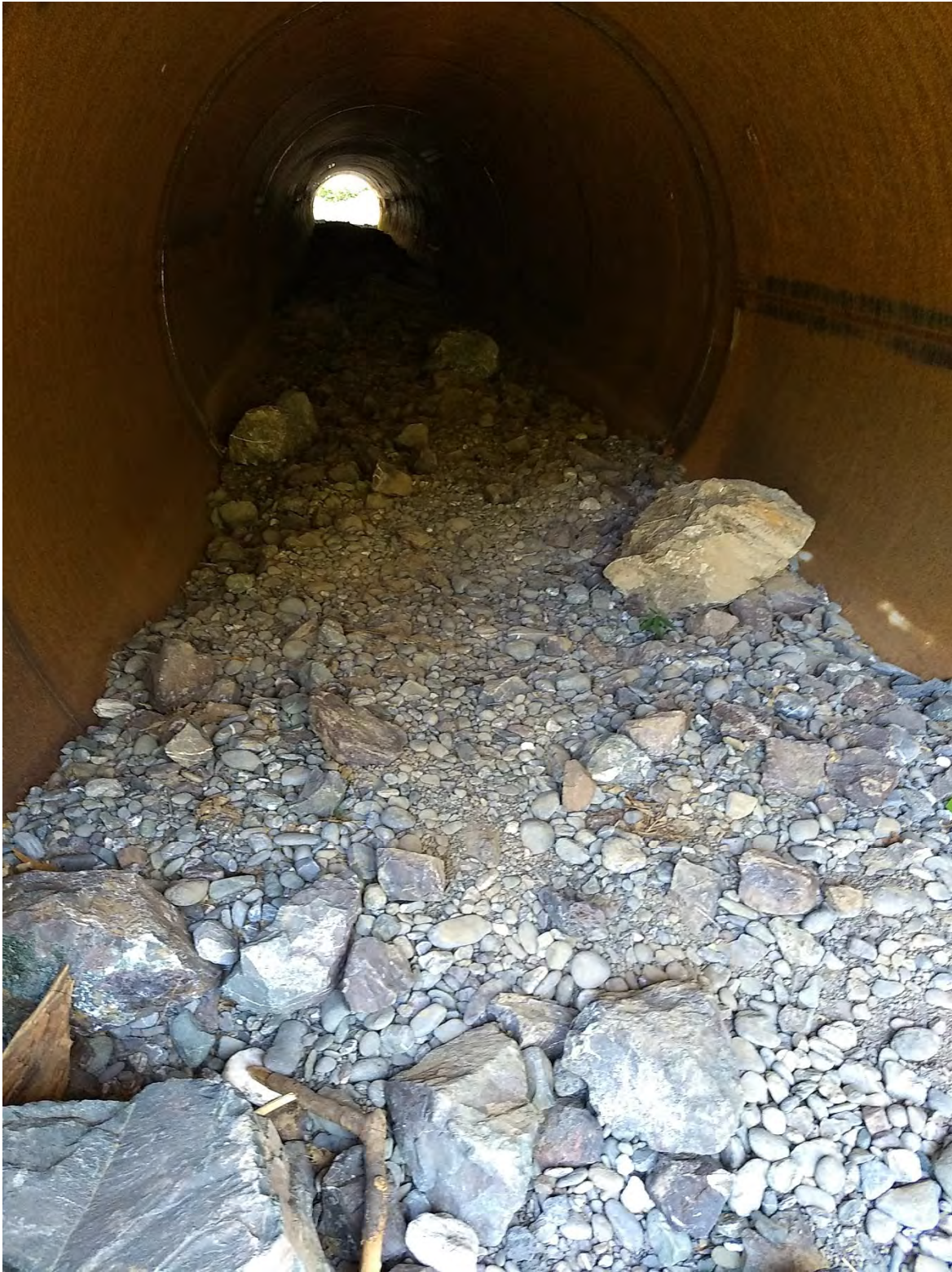
Figure 4. The higher culvert's invert and natural substrate bottom with keystone rocks looking downstream from the culvert inlet. Photo by Margaret Lang on 9/12/2019.
