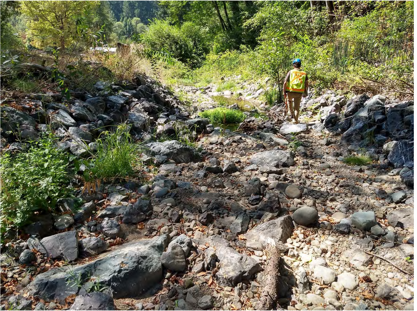
Figure 6. The downstream project channel looking downstream from the culvert outlet. Flow is discontinuous but surfaces behind most of the rock weirs. Photo by Margaret Lang on 9/12/2019.
