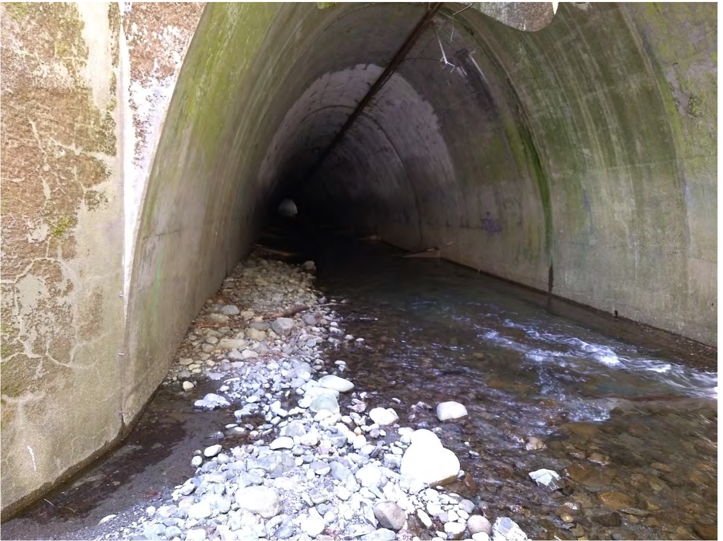
Figure 3. Cedar Creek culvert invert looking downstream from the inlet. The installed weirs are capturing sediment and maintaining a natural streambed near the inlet. Photo taken by M. Lang April 15, 2021.
