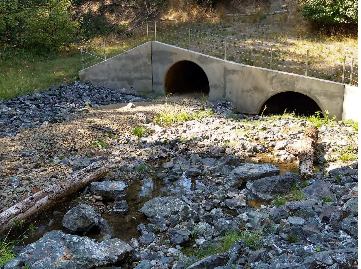
Figure 3. Close-up of the embedded inlets of the double-barrel South Fork Ryan Creek crossing. Photo by Margaret Lang on 9/12/2019.
