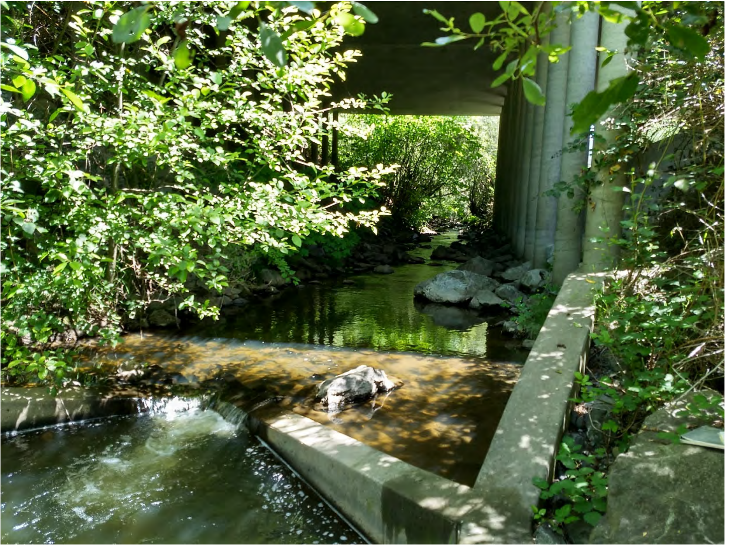
Figure 5. Hall Creek fish ladder looking upstream from the first weir to the natural channel bottom under the HUM 299 bridge. The ladder was installed to maintain the stream bed elevation at this upstream-most weir. Photo taken by M. Lang June 6, 2020.
