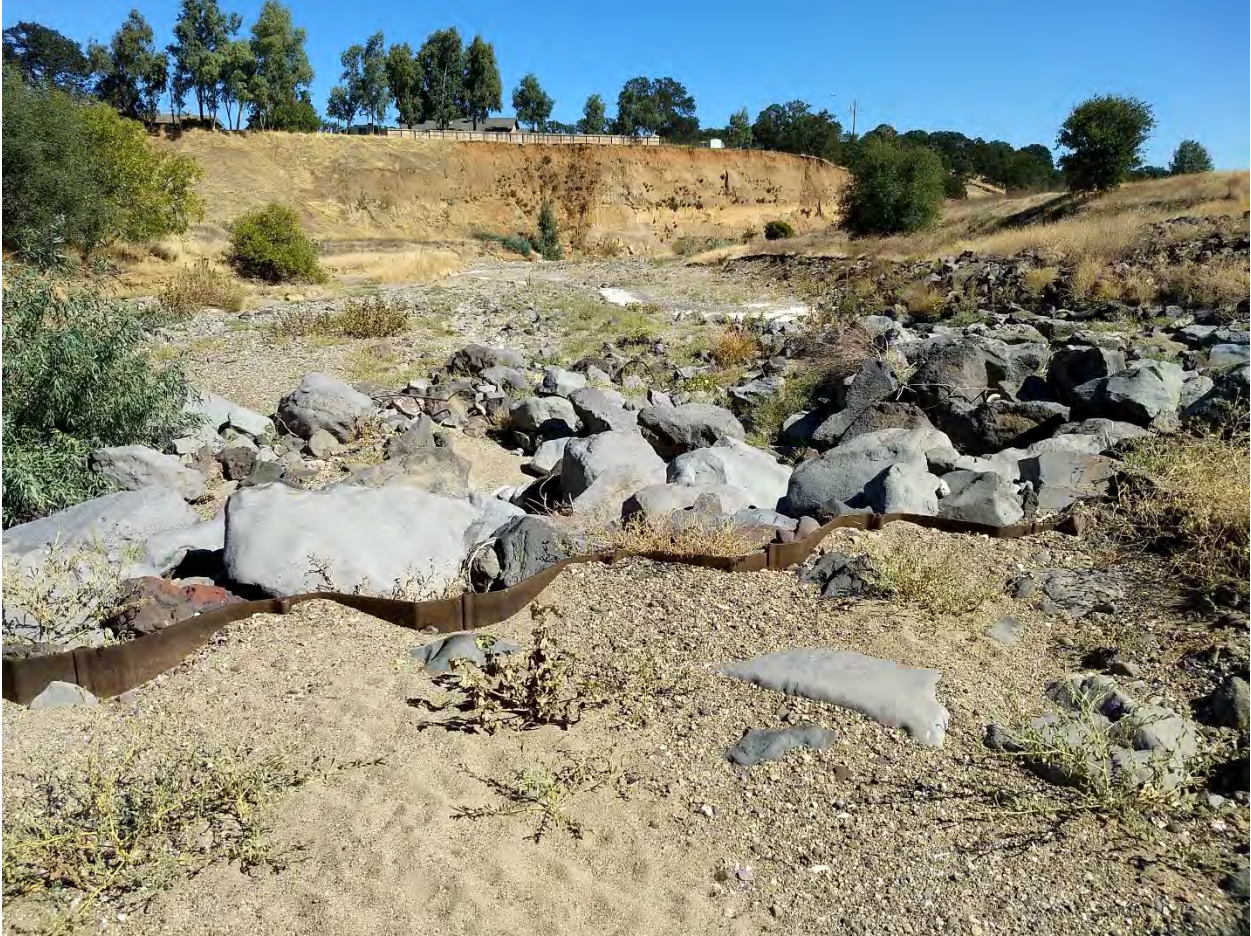
Figure 3. Dibble Creek looking downstream from the bridge left span. The low flow channel is on the right. The high rock weir in the picture forefront controls water elevation in the left channel to guide water to the low flow channel on the right. The sheet piling is just visible upstream of the rocks and is present but at lower creat elevation on both sides of the channel. Photo taken October 4, 2019.
