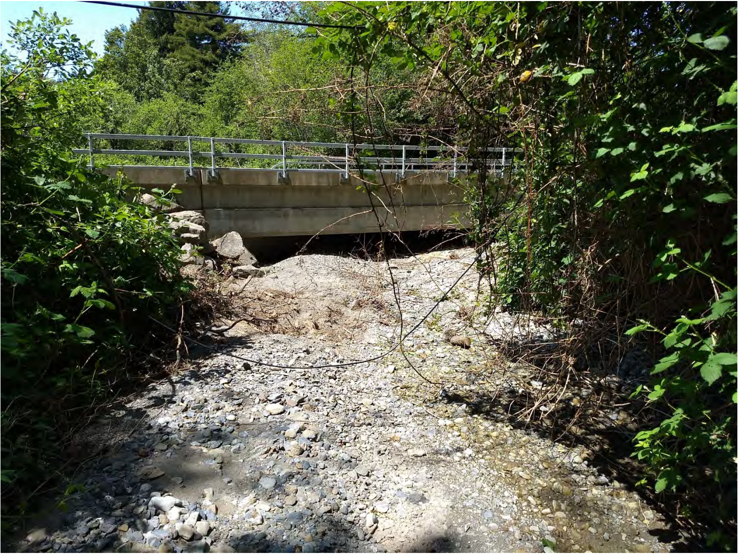
Figure 2. Sediment accumulation under the Sultan Creek bridge on Del Norte 197, postmile 5.00. View is looking downstream from the upstream channel.
