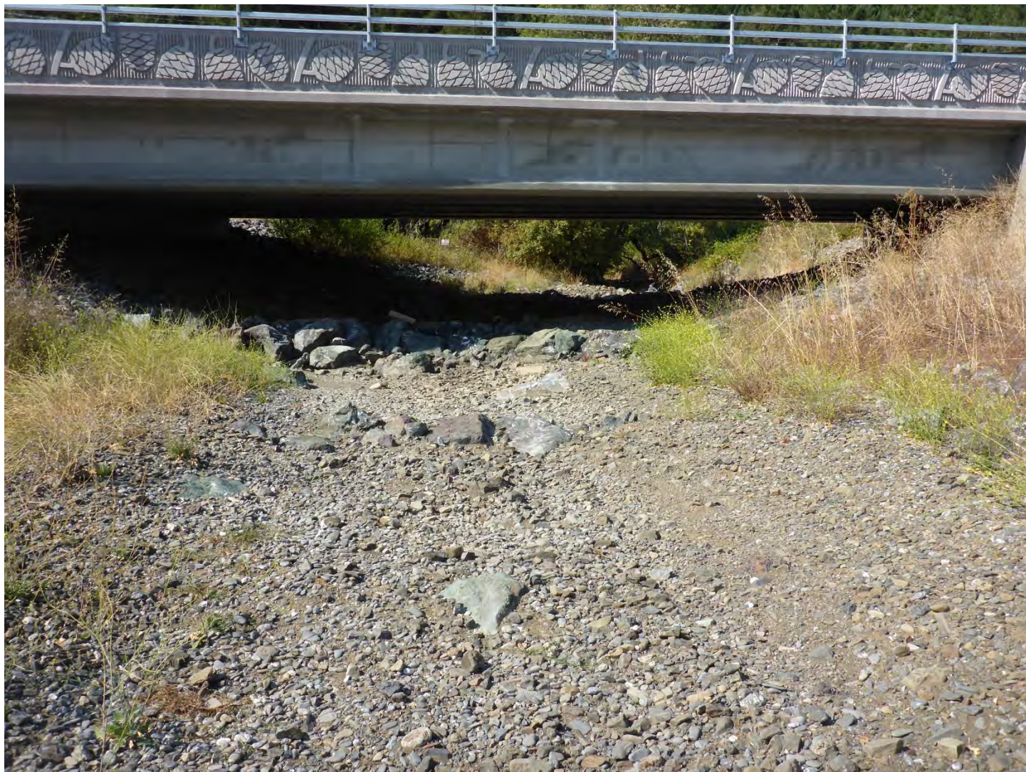
Figure 6. The weir just downstream of the bridge appear to be backwatered and being buried in sediment. Photo by Michael Love on 9/12/2019.
