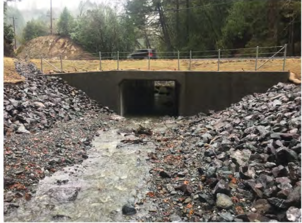
Looking Through Culvert at Inlet Post-Treatment. Photo taken on 01/09/2018 and courtesy of Caltrans.
