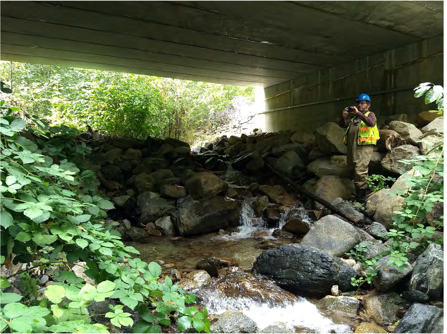
Figure 3. The channel bed under the bridge channel and transition into the downstream channel looking upstream. Photo by M. Lang on 9/19/2019.
