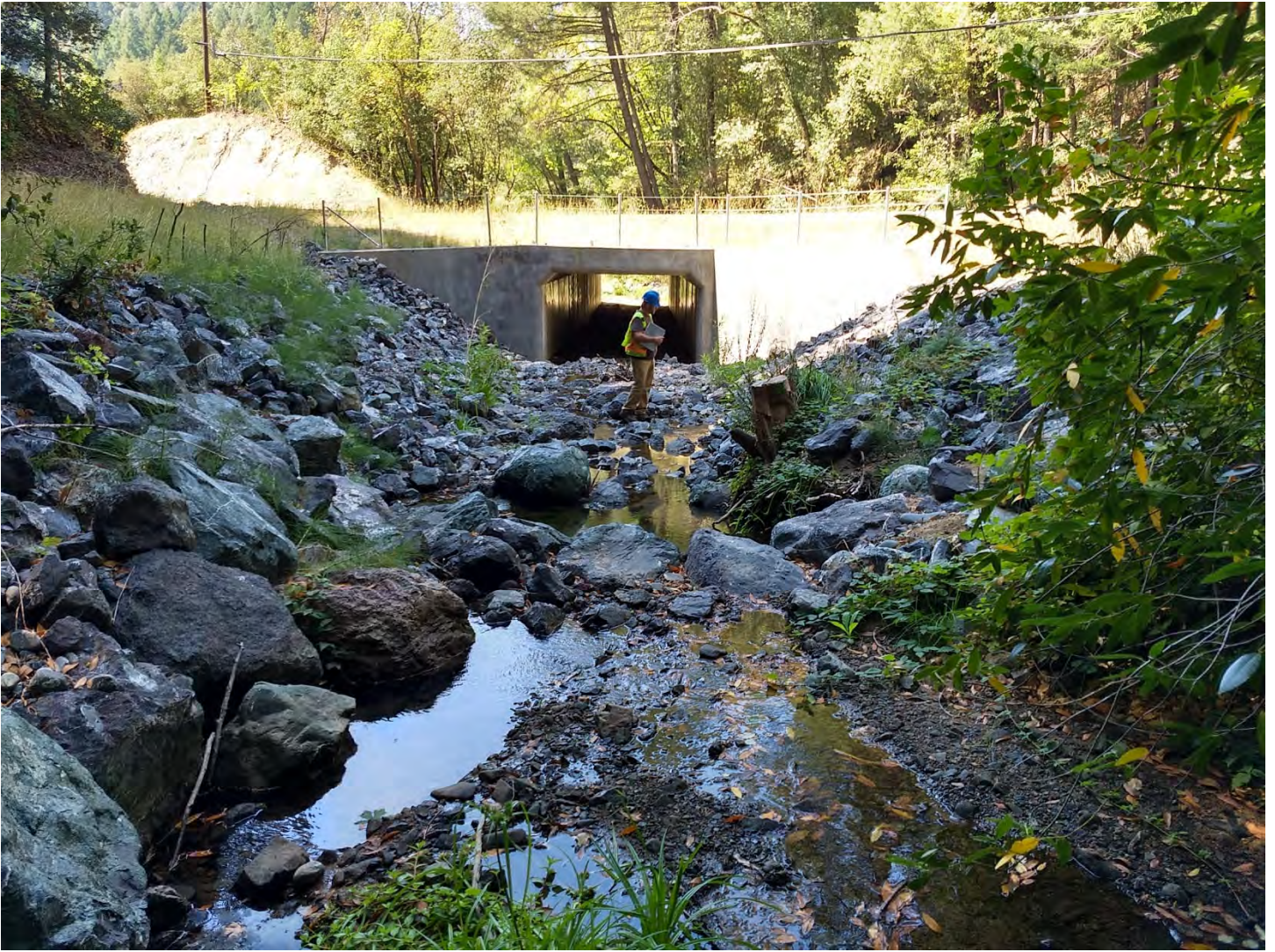
Figure 3. Culvert inlet looking downstream from the upstream project boundary. Stream flow was low but continuous upstream of the culvert during this site visit. Photo by Margaret Lang on 9/12/2019.
