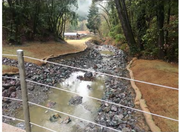
Downstream Post-Treatment. Photo taken on 01/09/2018 and courtesy of Caltrans.
