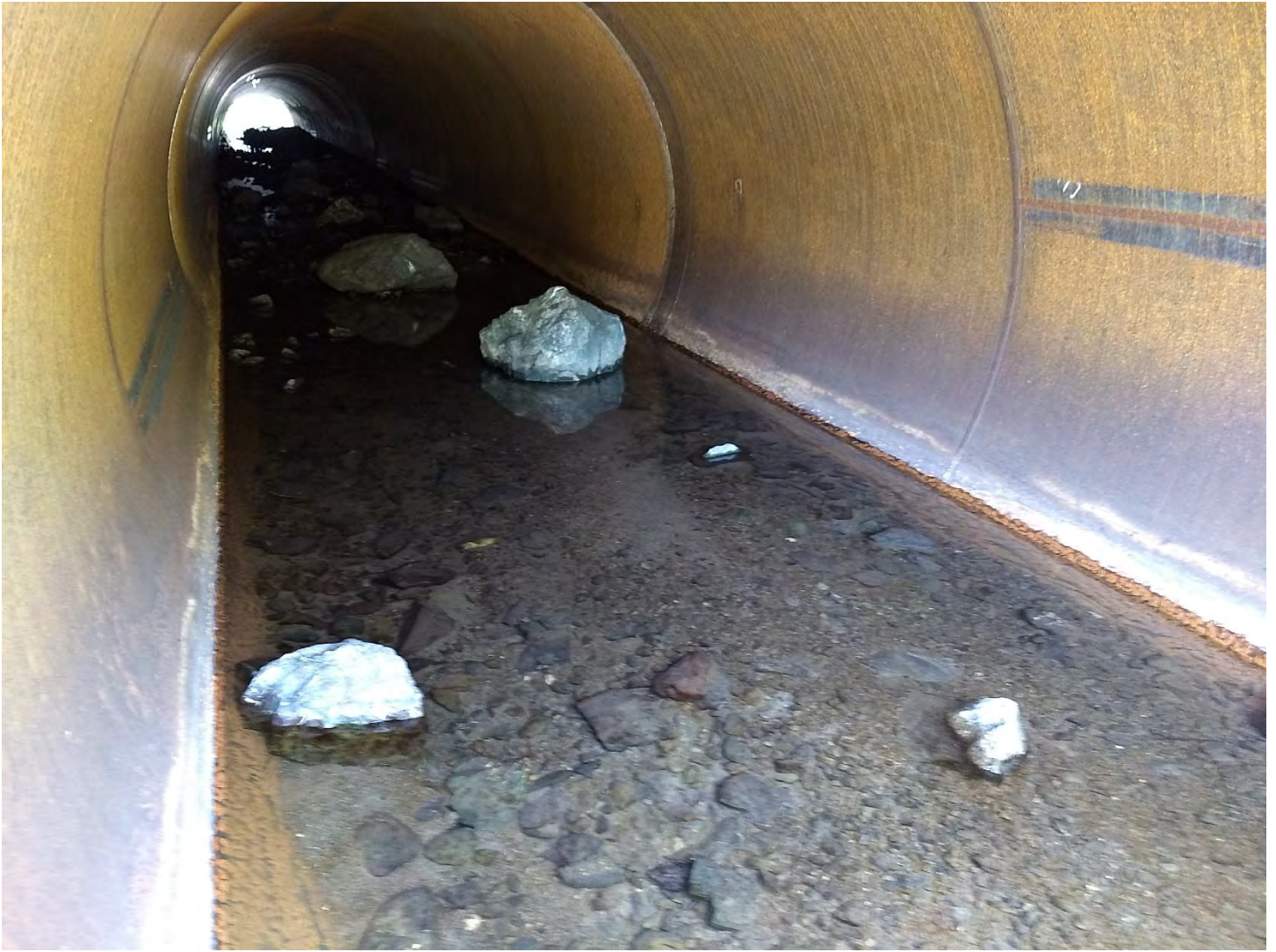
Figure 5. The lower culvert's invert and natural substrate bottom with keystone rocks looking downstream from the culvert inlet. Photo by Margaret Lang on 9/12/2019.
