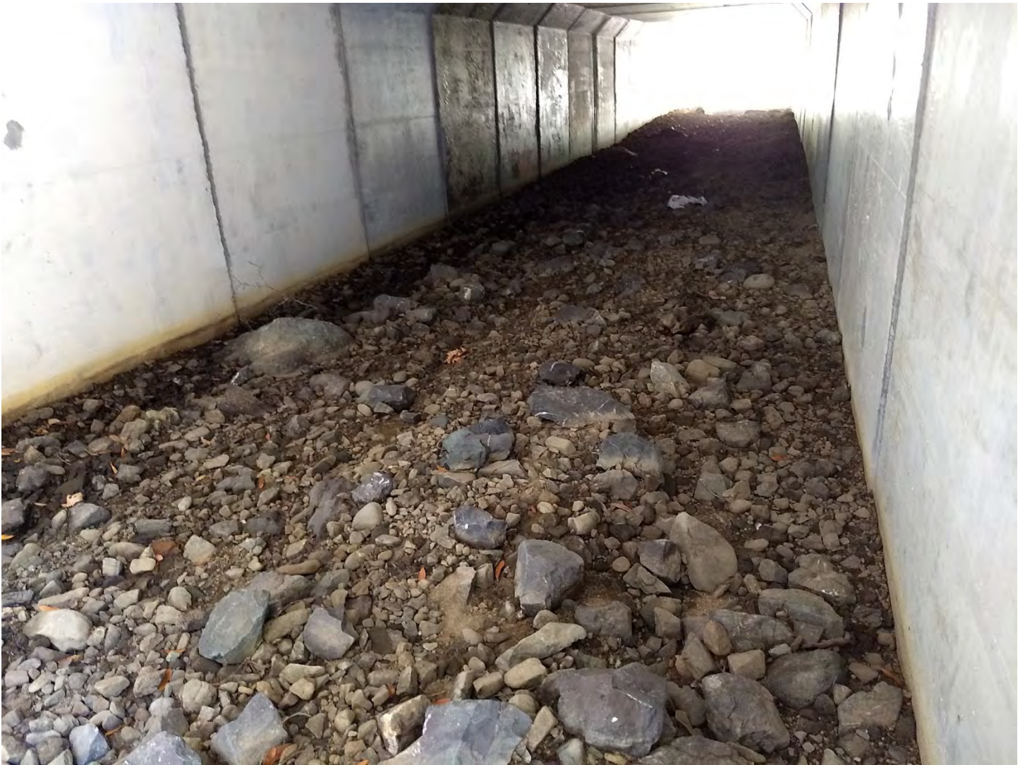
Figure 4. The culvert's invert and natural substrate bottom. The culvert substrate is almost a plain bed with the larger disruptor rocks mostly buried. At this low flow, there was no flow in the culvert, but it was very moist along the left side. Photo by Margaret Lang on 9/12/2019.
