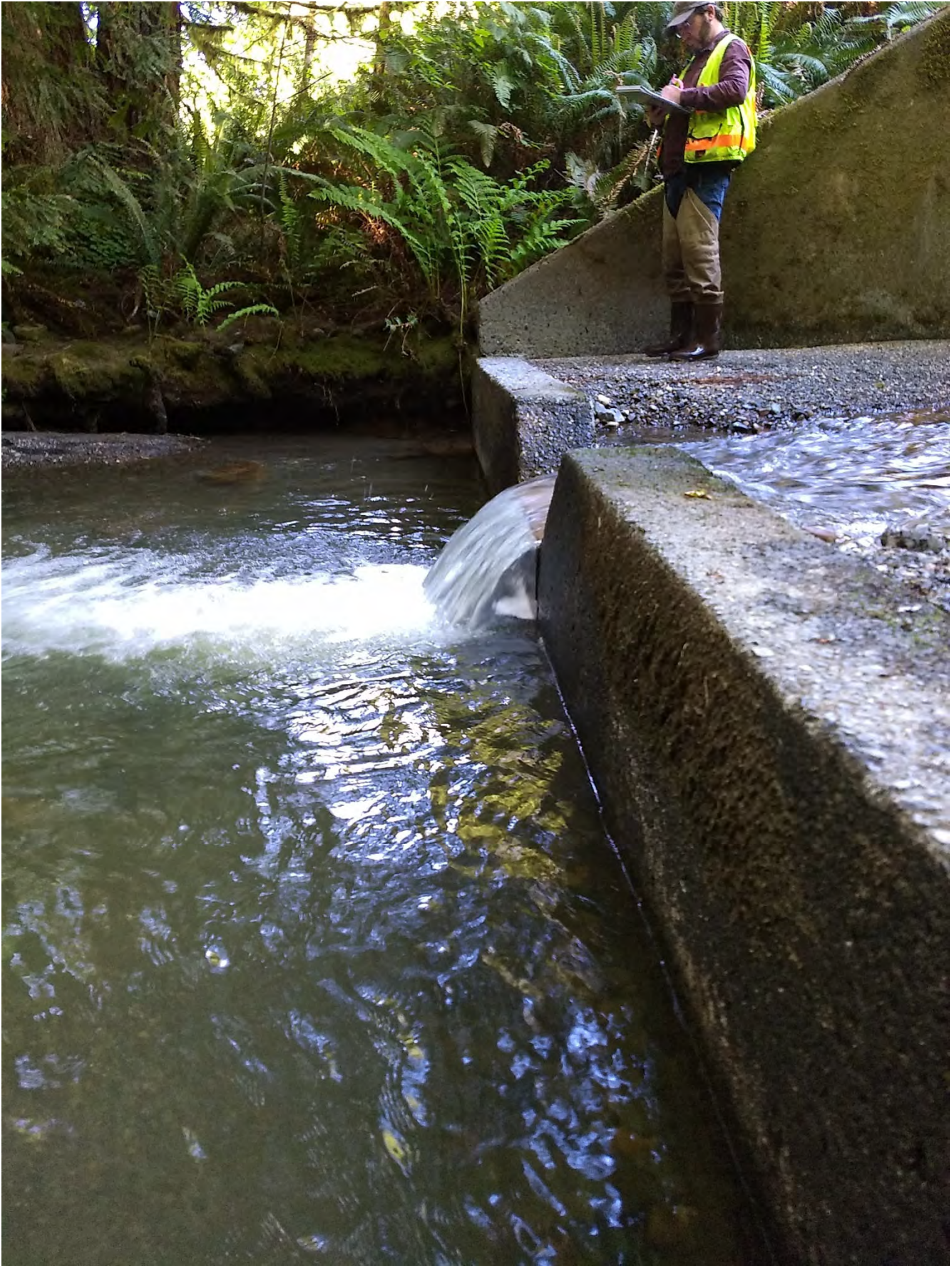
Figure 5. Concrete square-notched weir at outlet. Drop elevation is ~1 foot at low flow.
