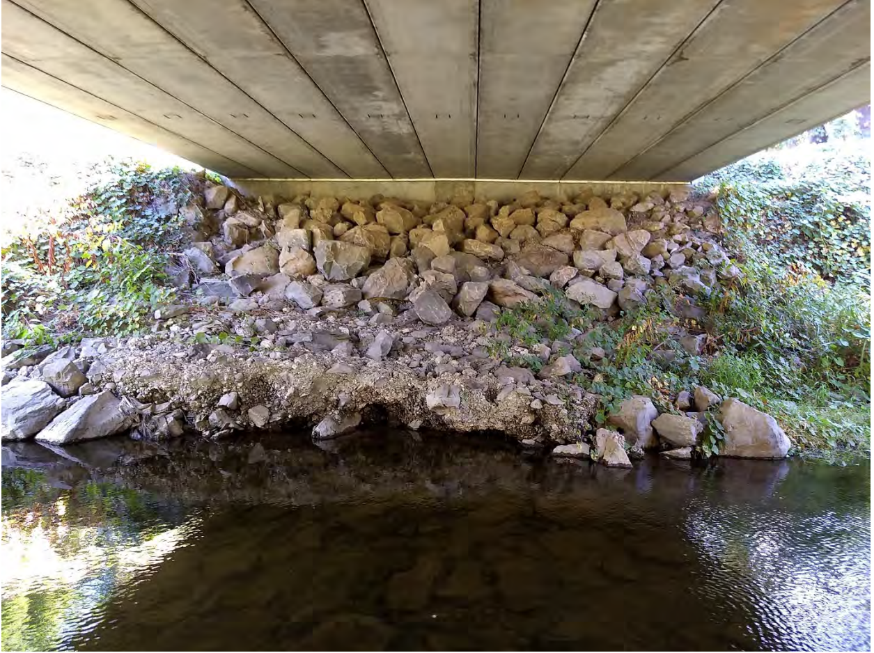
Figure 6. Craig Creek Right bank erosion and loss of bank protection by undercutting at the crossing. Photo taken October 4, 2019.
