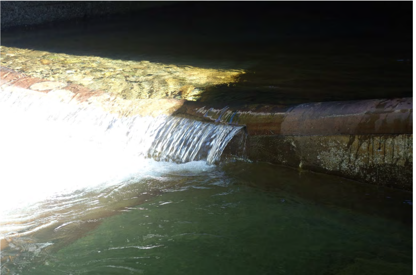
Figure 9. Cedar Creek culvert outlet weir. The concrete at this location has a small edge which was not smoothed out when the steel cover was installed. This edge creates a detached flow that does not wet the rounded section installed to assist lamprey migration. Photo taken June 3, 2021. (alternate view to supplement Figure 8)
