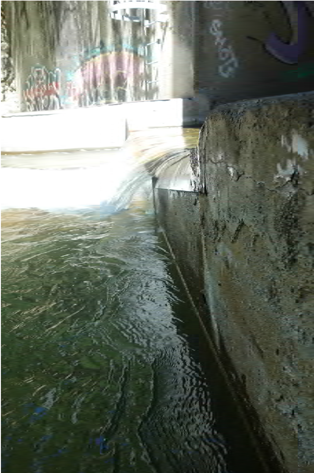
Figure 8. Cedar Creek culvert outlet weir. The concrete at this location has a small edge which was not smoothed out when the steel cover was installed. This edge creates a detached flow that does not wet the rounded section installed to assist lamprey migration. Photo taken June 3, 2021.
