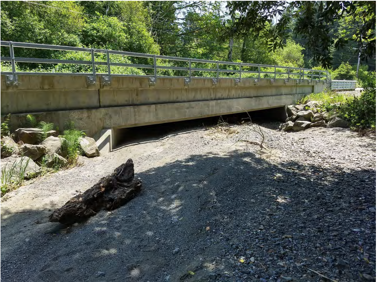
Figure 1. Sediment accumulation under the Sultan Creek bridge on Del Norte 197, postmile 5.00. View is looking upstream from the downstream channel.
