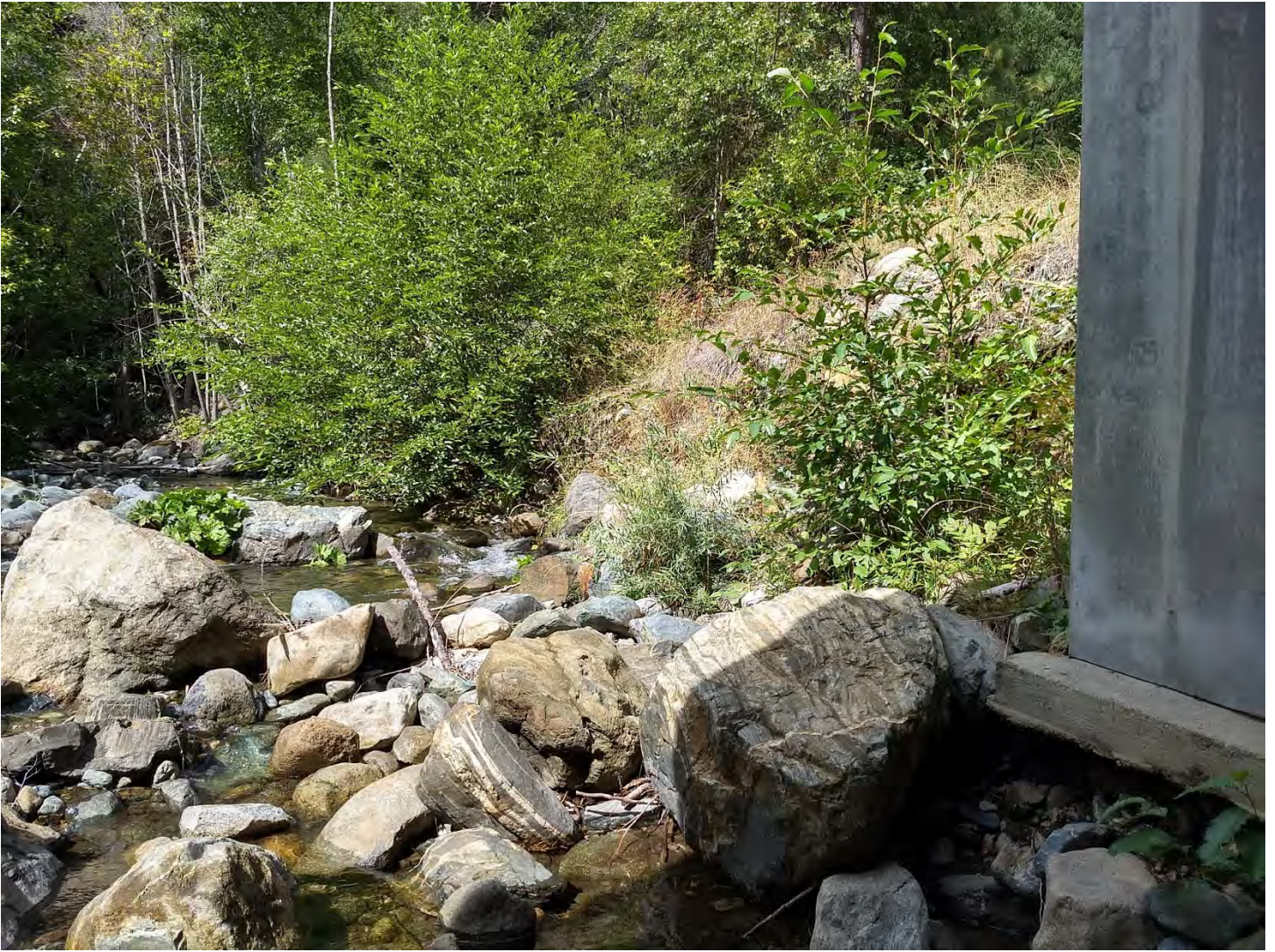
Figure 5. Upstream, left bank and bridge footing showing scoured bank protection and exposed footing. This is an outer channel bend coming into the bridge project site. Photo by M. Lang on 9/19/2019.
