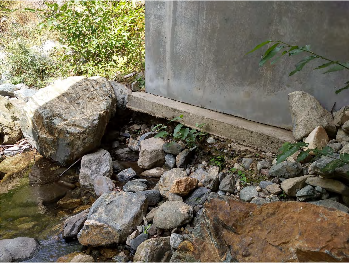
Figure 4. Close-up of upstream, left bank of bridge showing scoured bank protection and exposed footing. Photo by M. Lang on 9/19/2019.
